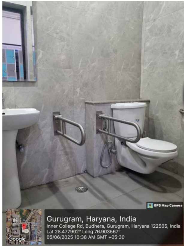
Accessible toilet with fold-up grab bars and hand shower
